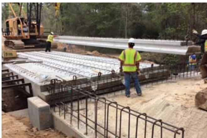
Precast concrete beams being placed for bridge construction on Black Oak Drive
